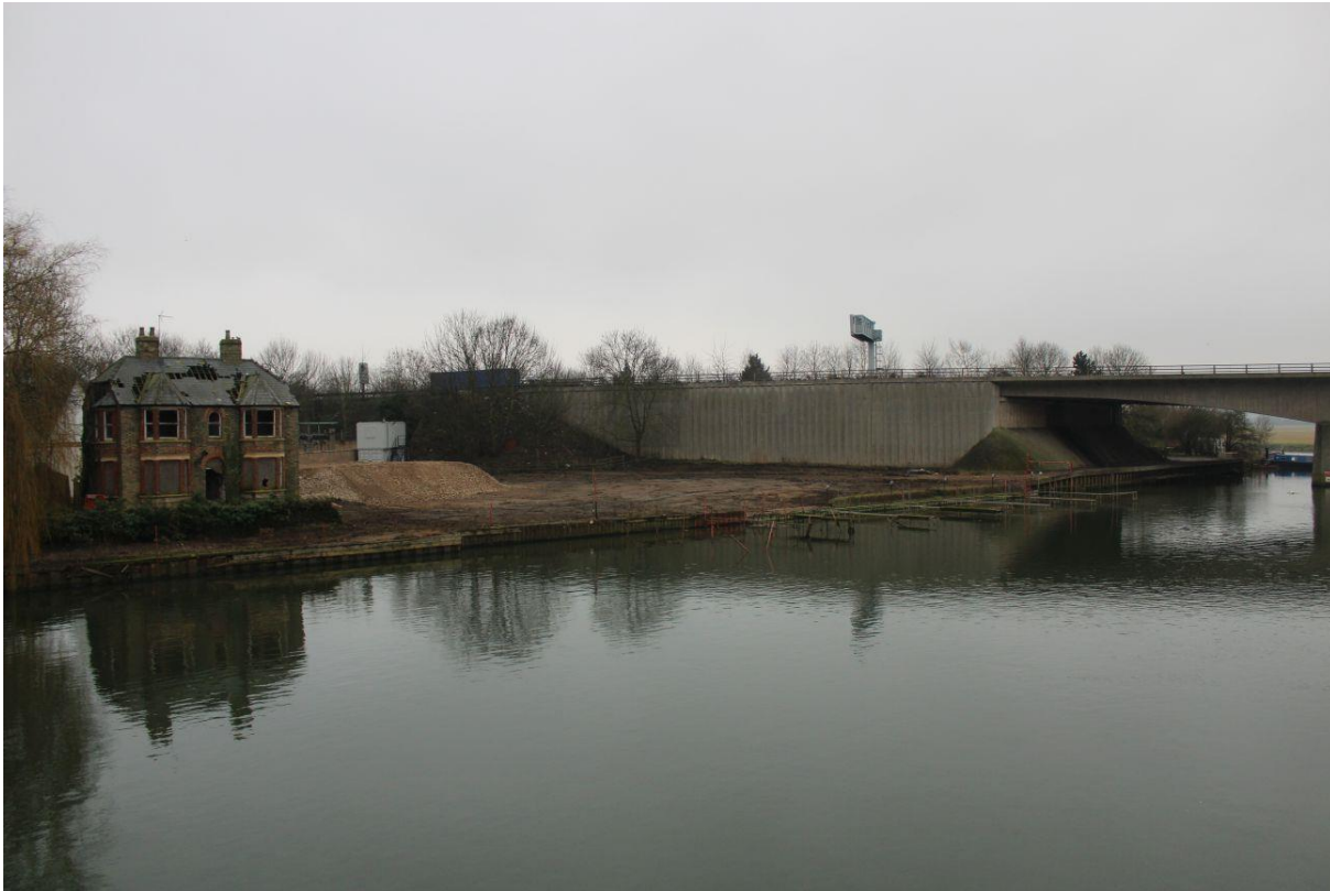
Figure 9: Construction site adjacent to the River Great Ouse, Huntingdon. (Source: Ben Clifford, 2017)
