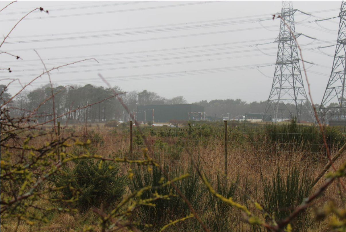
Figure 23: The Galloper sub-station under construction, as seen from the road in February 2017. (Source: Ben Clifford, 2017)
