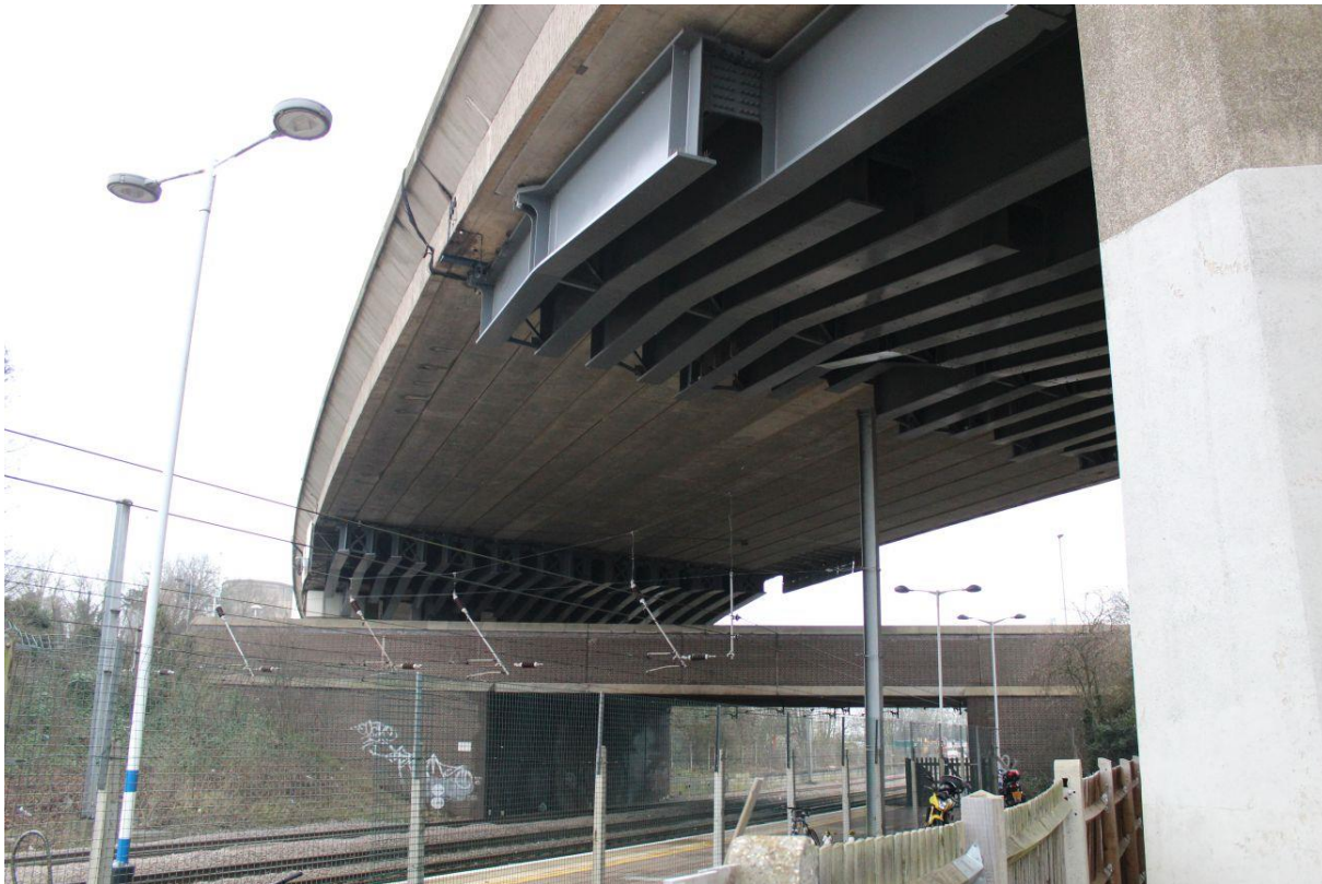
Figure 11: A14 flyover over local road and the East Coast Mainline at Huntingdon Station. (Source: Ben Clifford, 2017)
