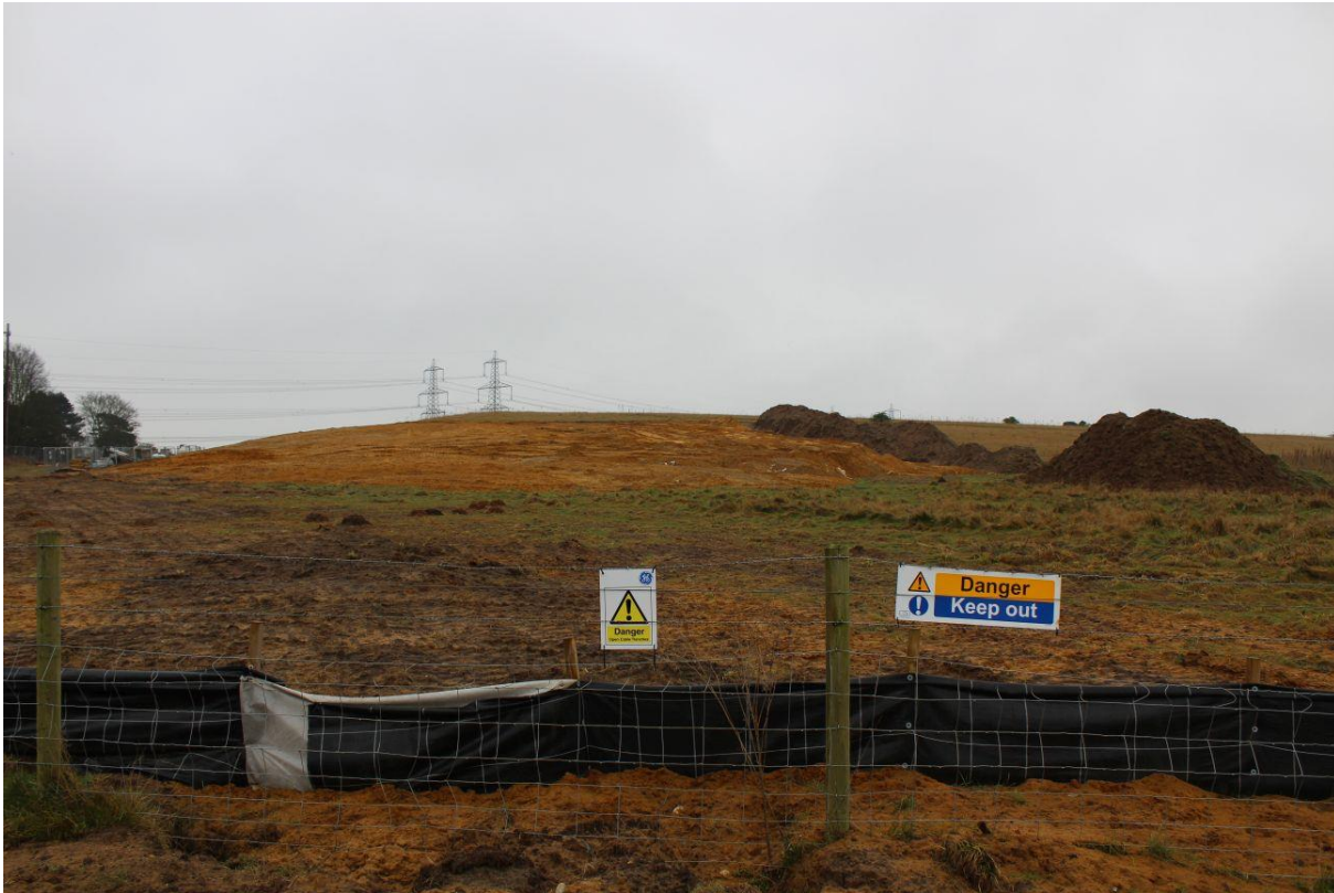
Figure 21: Construction of an earth mound as visual mitigation at Galloper sub-station. (Source: Ben Clifford, 2017)
