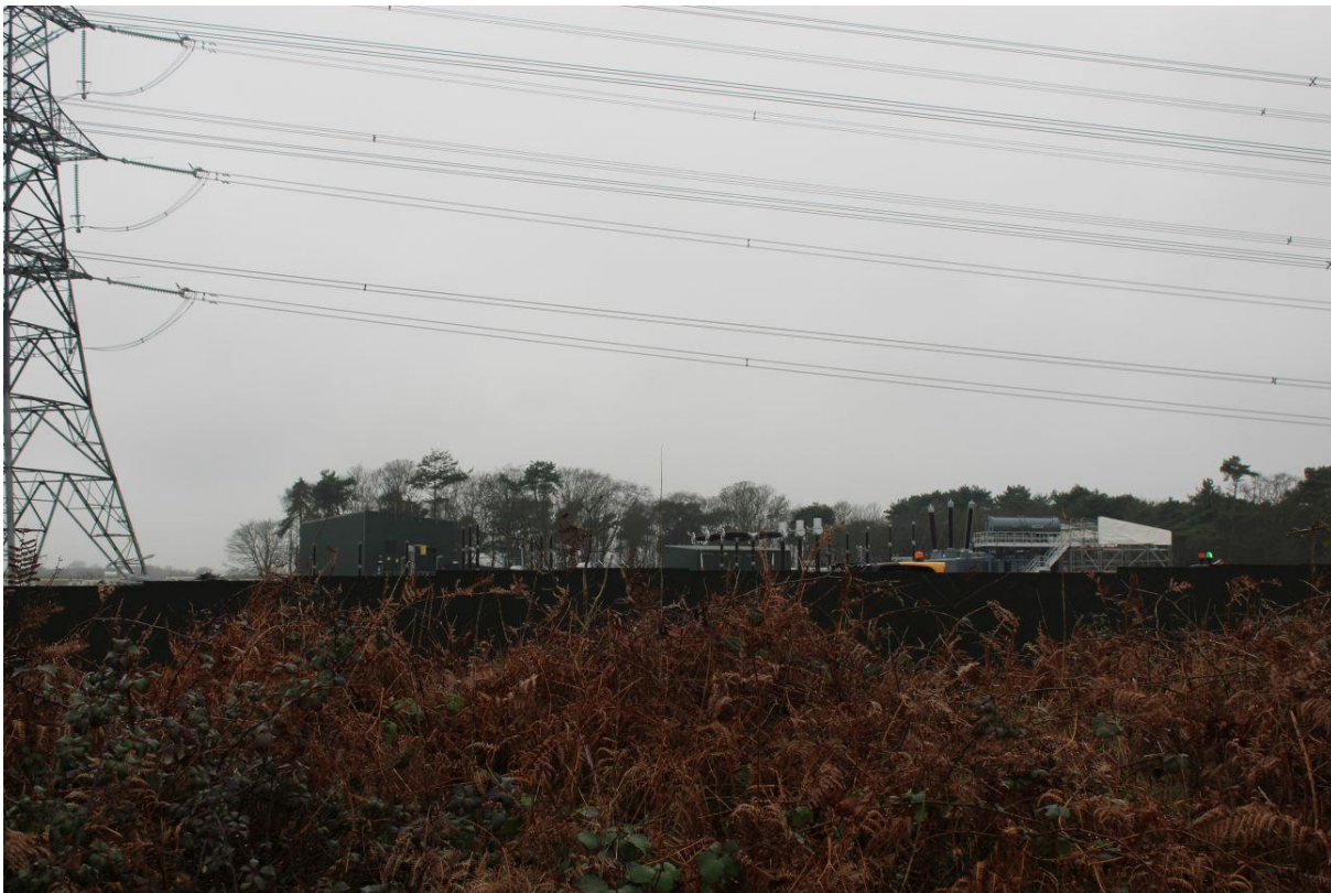
Figure 20: The sub-station for the Galloper offshore windfarm, Sizewell. (Source: Ben Clifford, 2017)
